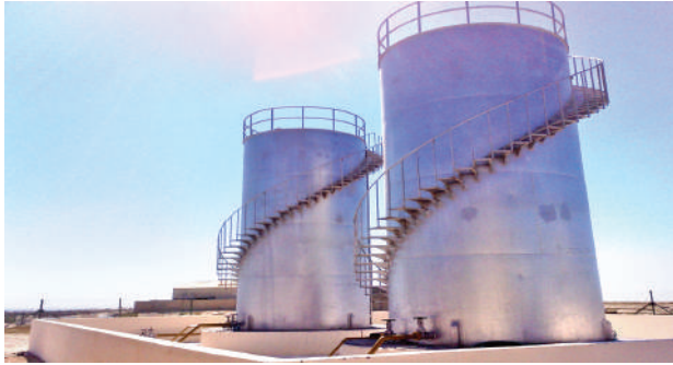
FUEL STORAGE TANK
